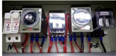
Gambar 14. ATS Automatic transfer switch
