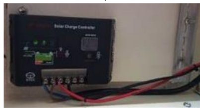
Gambar 18. pengujian Control Charger
