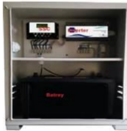
Gambar 13 Panel Box listrik Hybrid
