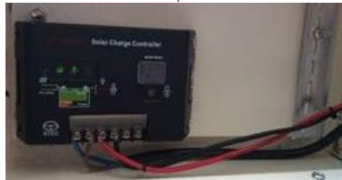
Gambar 18. pengujian Control Charger
