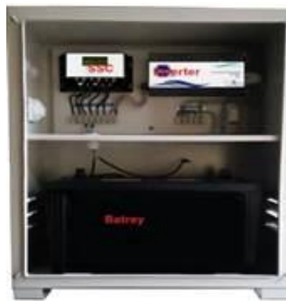
Gambar 13 Panel Box listrik Hybrid
