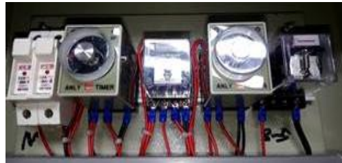
Gambar 14. ATS Automatic transfer switch
